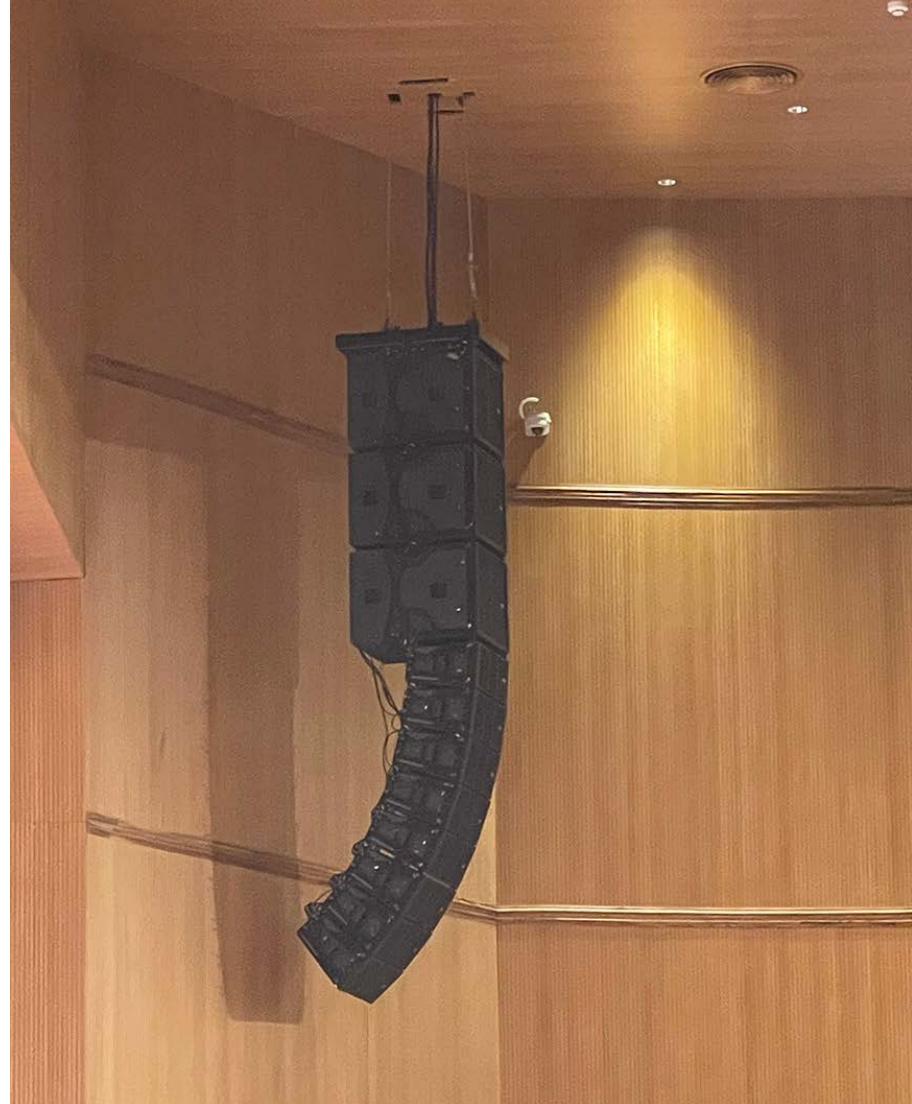
The self-powered line array system from AUDIOFOCUS completes the pro audio install at the Veronica Auditorium, promising an unrivalled audio experience for the audience
